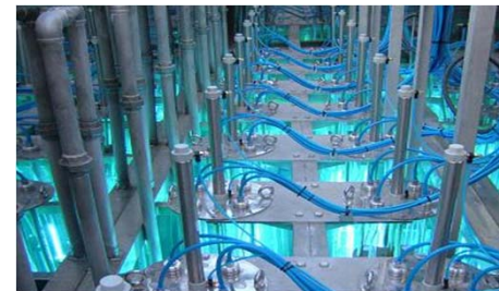
UV Disinfection for safe, potable water
